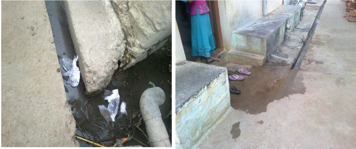
Drainage in Siddhapur village of Bilgi Taluk(Narrow Drain causing water logging)
