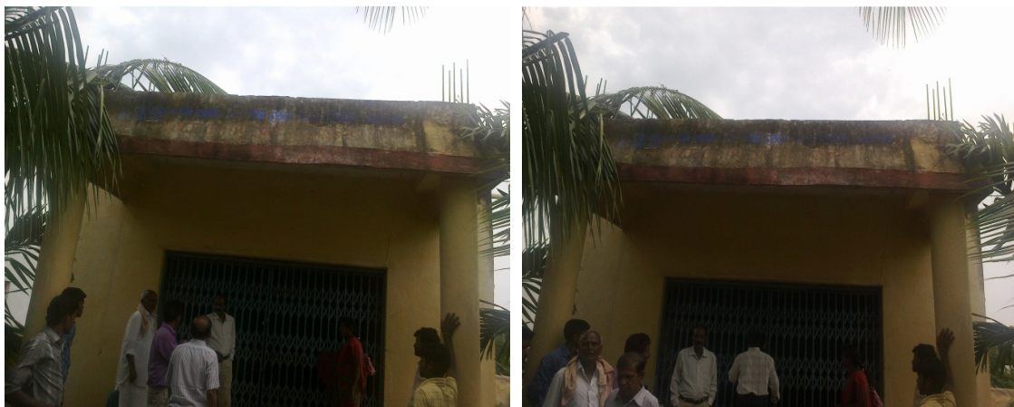
Samudaya Bhavan in Devgiri Village of Haveri Taluk(Incomplete doors windows&roof)
